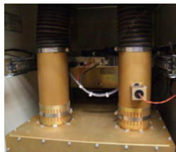
Burn Hazard, pipes over 220C
